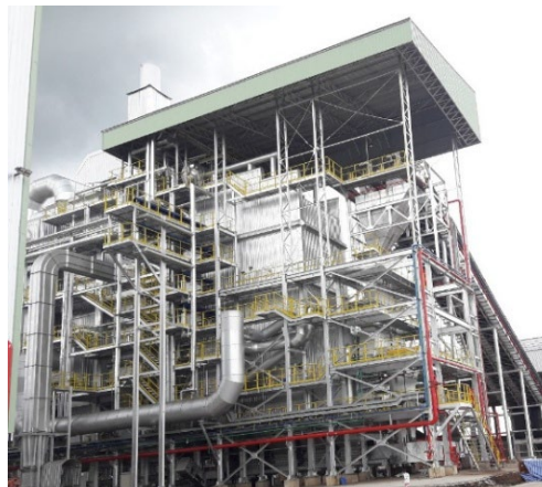
Figure 2. Incineration furnace and steam boiler building of a waste-to-energy power plant
