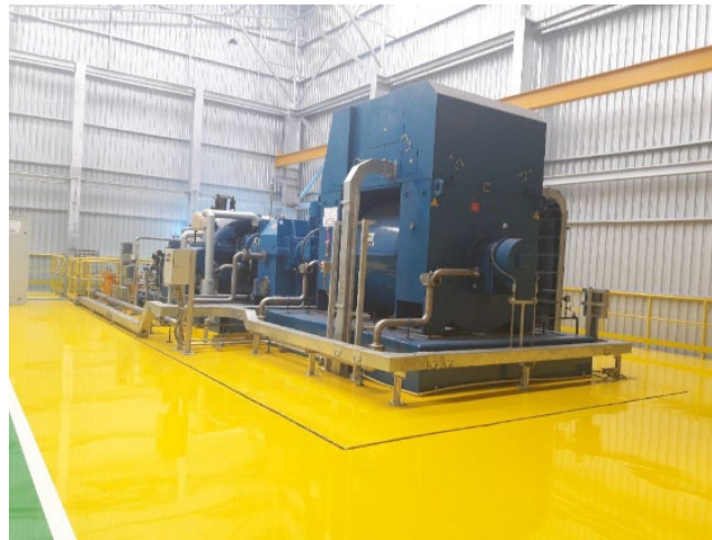
Figure 3. Steam turbine and electric generator units used for converting thermal energy from high-pressure steam into electrical power
